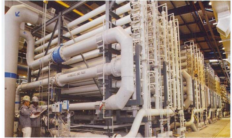
Fuairah Water & Power Plant
